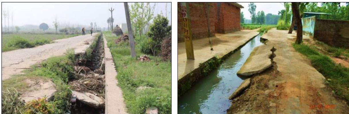
Fig. 3.2: Breakage in Gadarjudda minor
