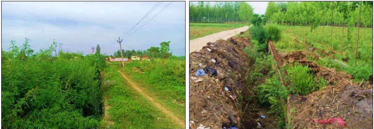
Fig. 3.3: Extensive weeds and vegetation in the canal
