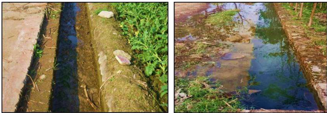
Fig. 3.8: Siltation in watercourse and overtopping due to siltation
